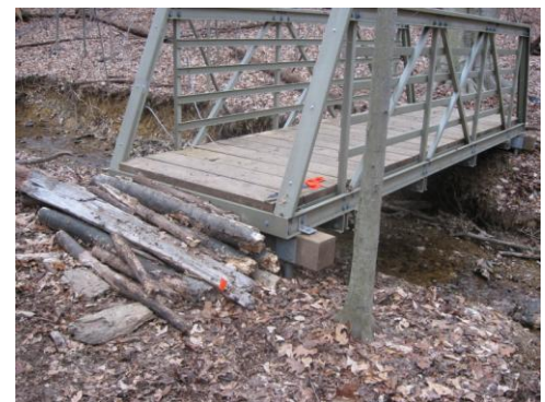
Bridge in need of an approach ramp
